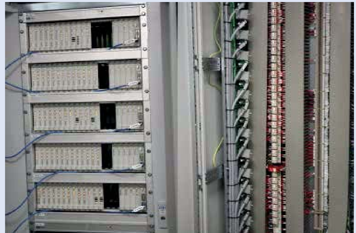
Typical Laser Controlled Area conduit
